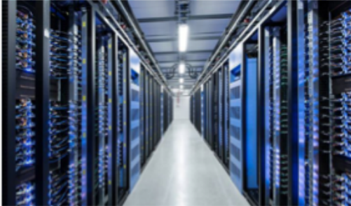
Data center optimization
